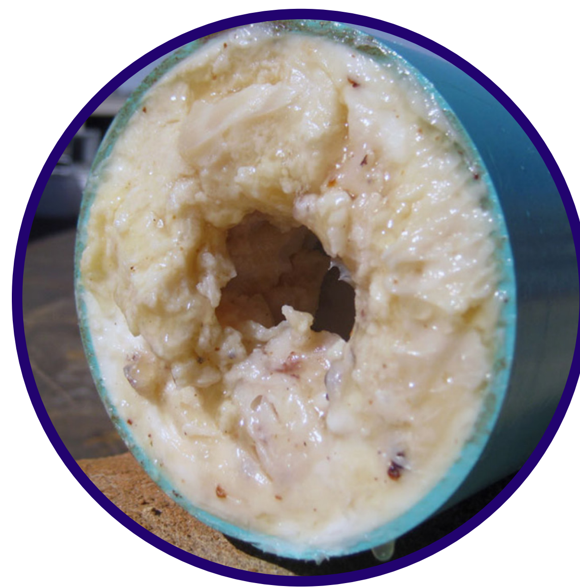
Fats, Oil, and Grease (FOG) clog up sewer pipes. Credit: 2017 Arlington County Government
