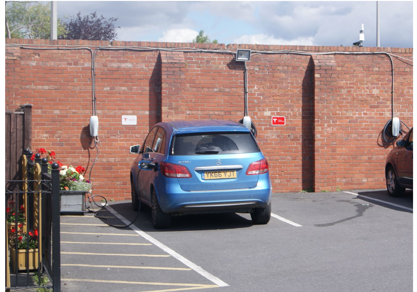
Electric car charging in parking lot in West Yorkshire. MTAYLOR848
