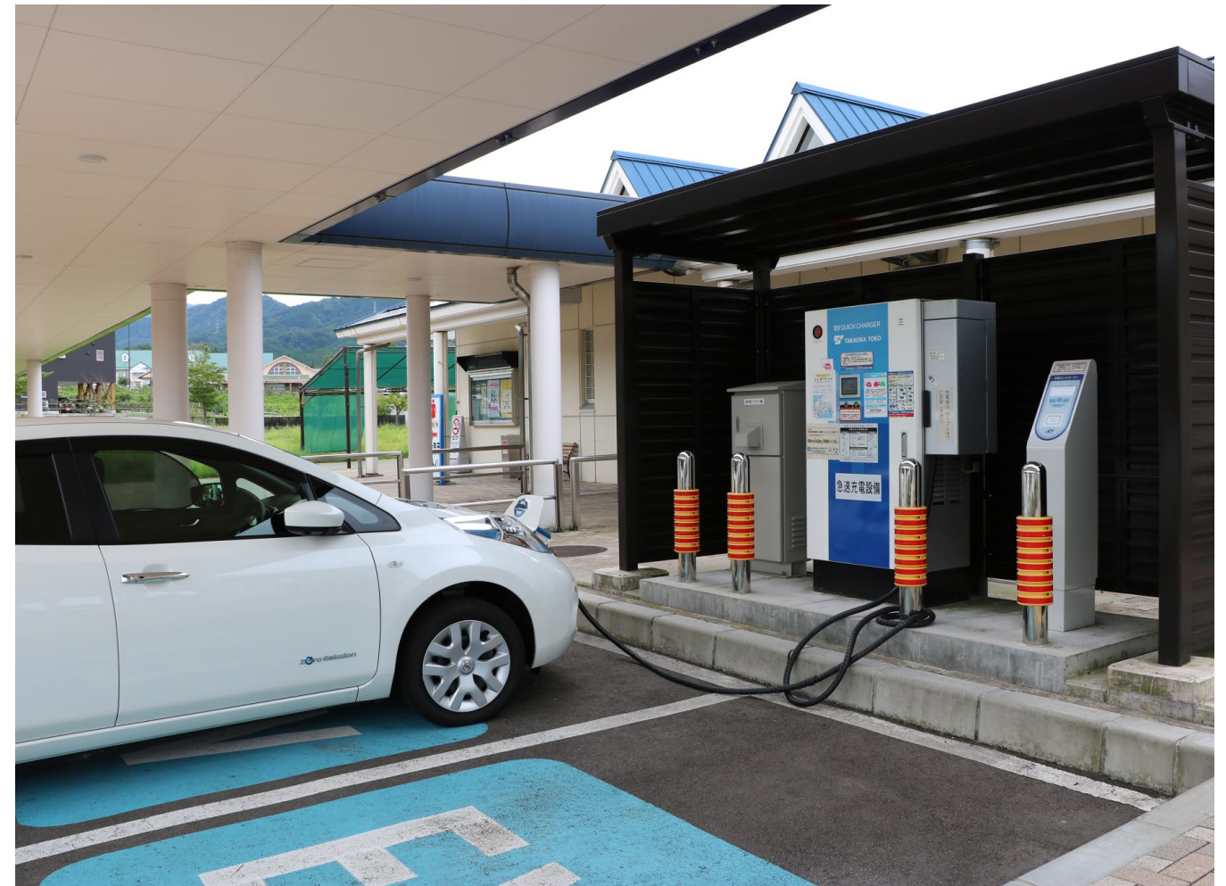
Constructing public charging stations is important for overcoming range limitations and for promoting use of electric vehicles. さかおり
