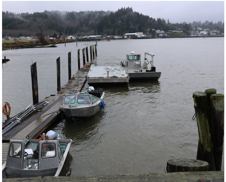
Figure 18: Current dock condition
